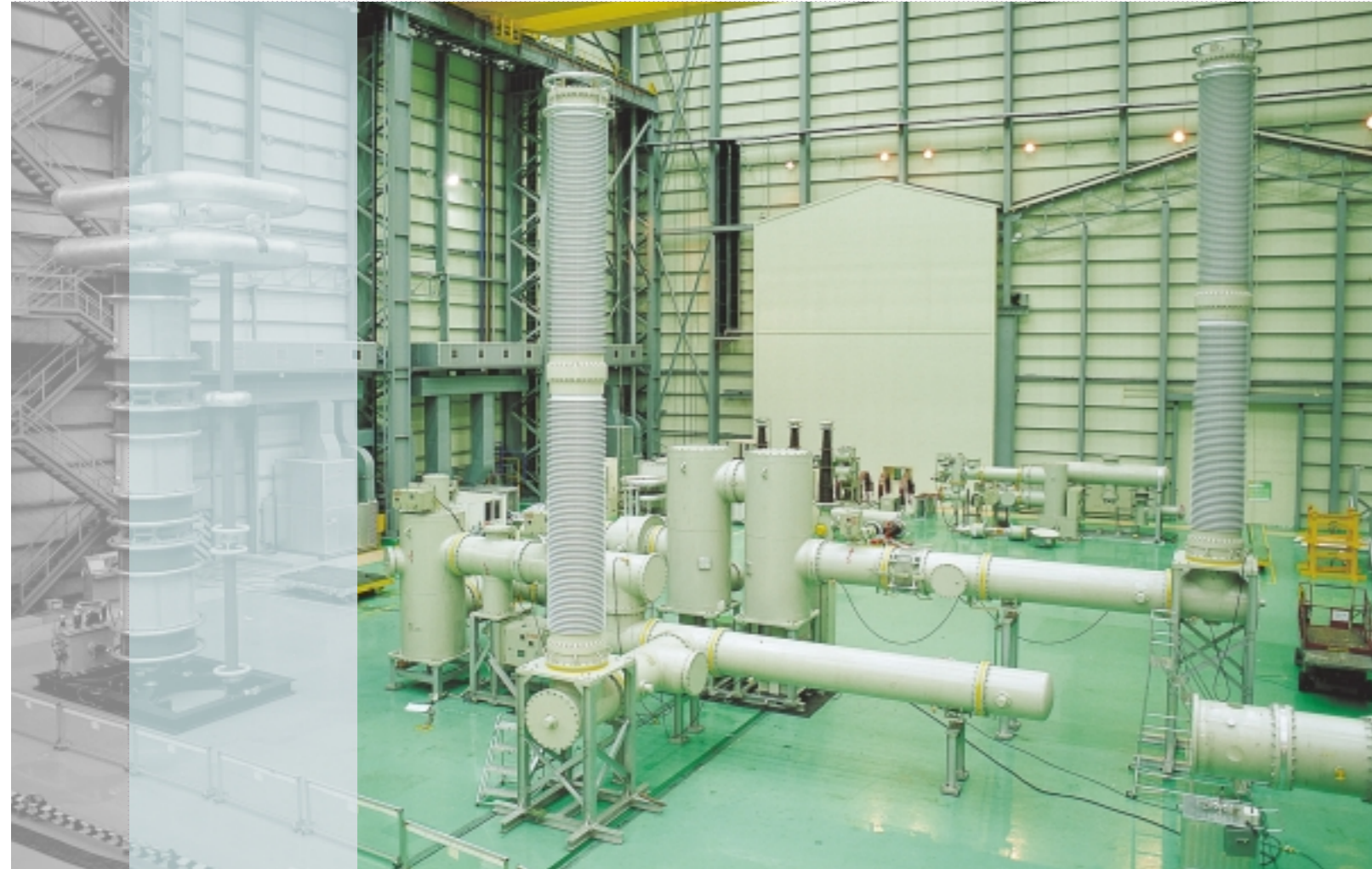
Gas Insulated Switchgear
