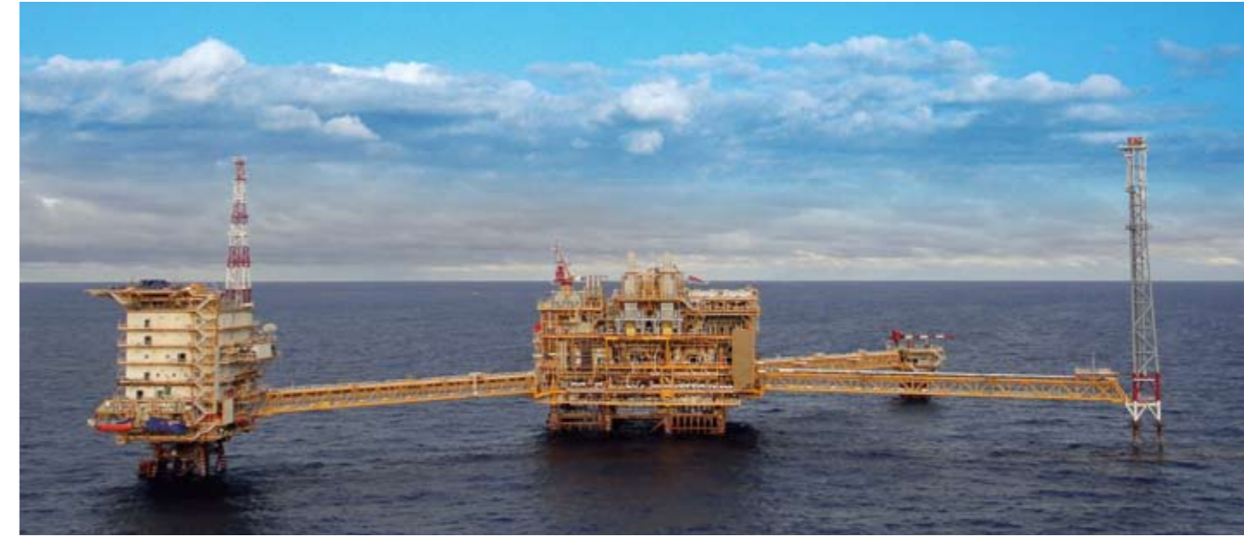
Bongkot South platform installation In August 2011, we installed this 30,000-ton processing platform for PTT Exploration and Production of Thailand. Designed to process 385 million square cubic feet of natural gas and 15,000 barrels of condensate per day, the platform is now operating in the Great Bongkot South field, 600 km southeast of Bangkok.
