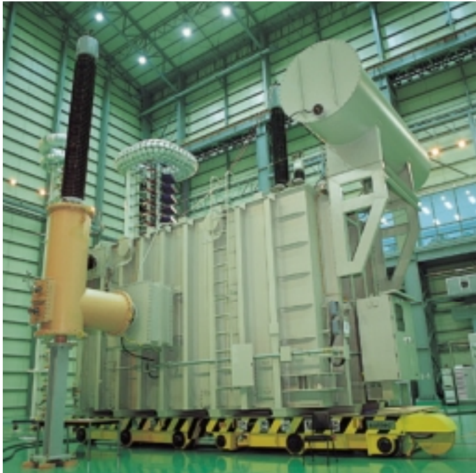
Power Transformer / 765kV
